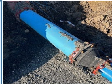
Distribution System Flushing
