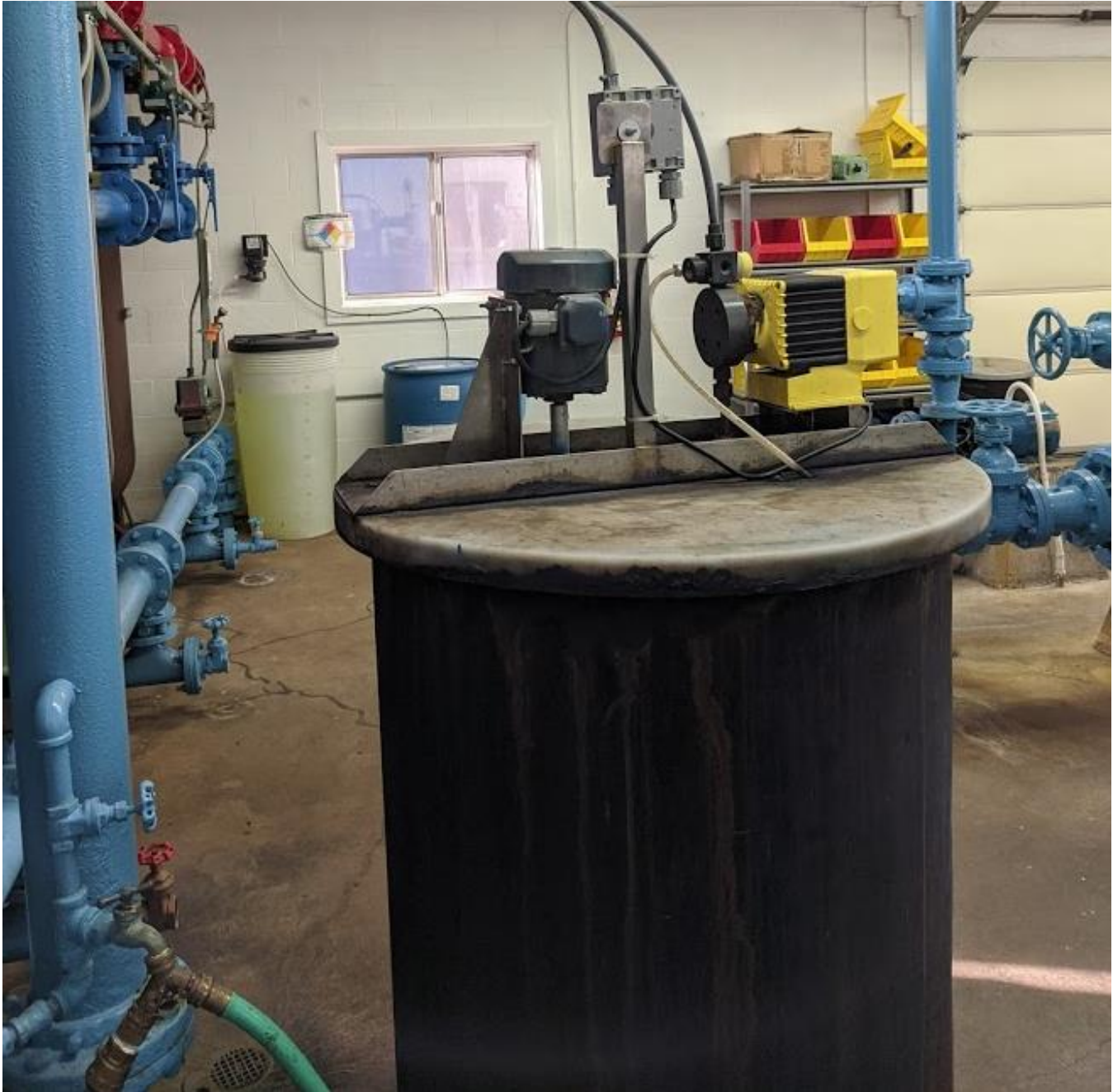
Figure V-2. Existing Potassium Permanganate Chemical Feed System
