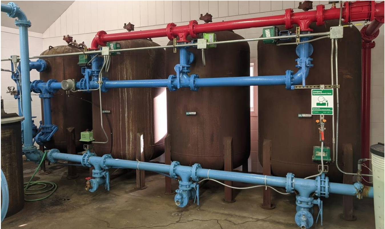
Figure V-1. Existing Pressurized Green Sand Filter System
