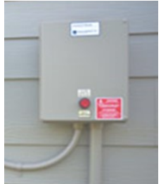
Sewer Alarm Box
