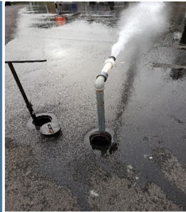
Distribution System Flushing
